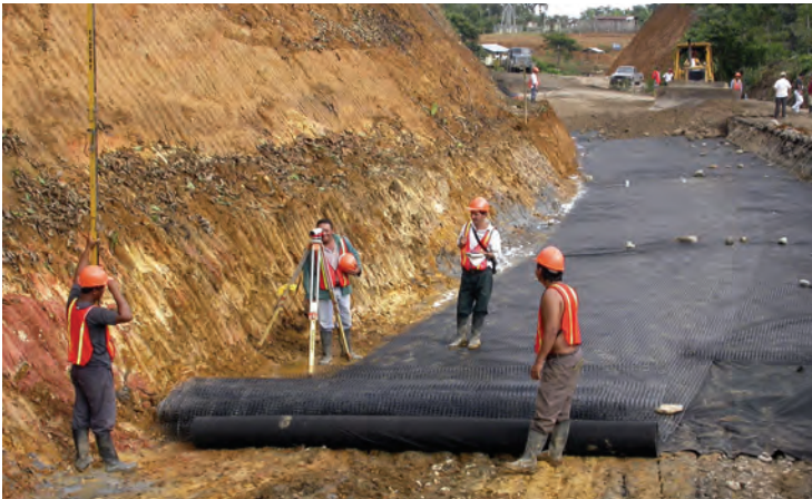
BASF's light stabilizers from the Chimassorb® range have been used by Megaplast India Pvt. Ltd., a leading polyethylene products manufacturer in India to produce nonwoven geotextile used in the construction of national highways.
